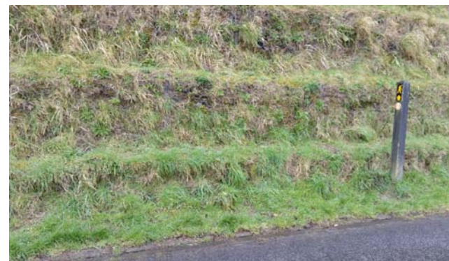
Green retaining walls where required – gabions over grown with local herbaceous/grassy vegetation
