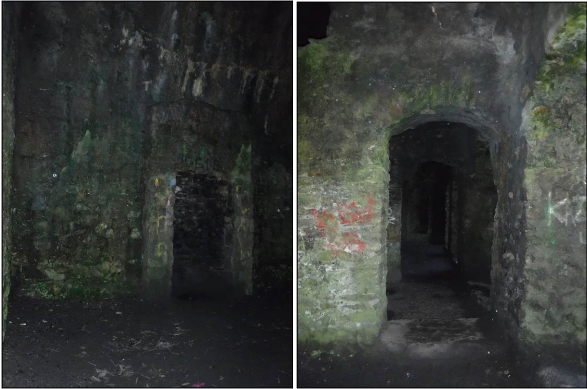
Figure 12.14 (Right) View looking west from the east room on the first floor. Note the changes in level at the door
