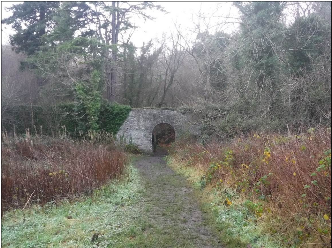
Figure 12.27 Arched entrance in the west wall of the formal garden. Note the fissure in the wall above the arch
