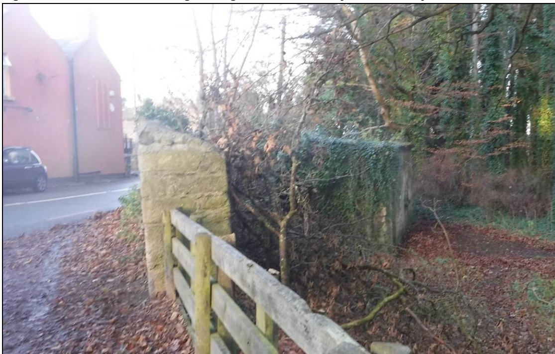
Figure 12.41 South wall of the gate lodge and the boundary wall to Massy's Wood
