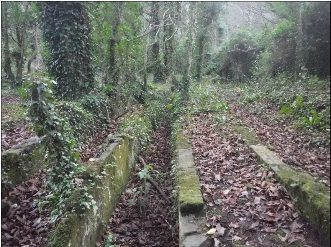
Figure 12.33 Brick foundations of some of the glass houses. Services ran in between the brick walls
